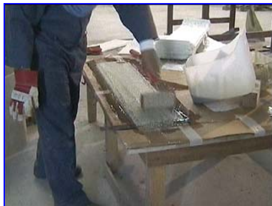
Impregnation of the laminate "pack" for pre-lamination of the PVC fitting. The purpose of this pre-lamination is to insure
