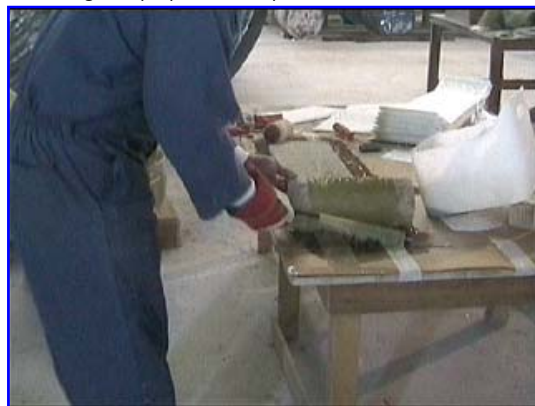
uniform bonding all throughout the surface of the PVC fitting, which is otherwise difficult to visually
